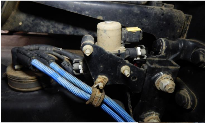
DEF lines going from tank to dosing unit. Blue Lines (universal).
